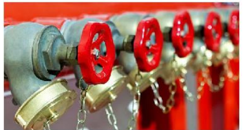
MODERN FIRE FIGHTING SYSTEM
